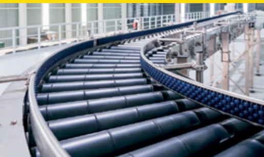
Controls the conveyor system throughout the production
